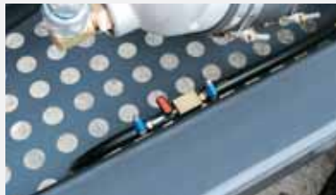
Fuel tank water drainage cock
