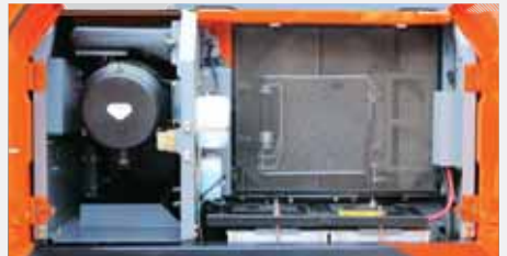
Utility space and radiators
